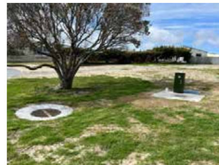
Pump station Darroch Slope
