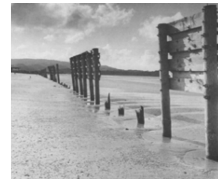
Little of the wall was left standing
